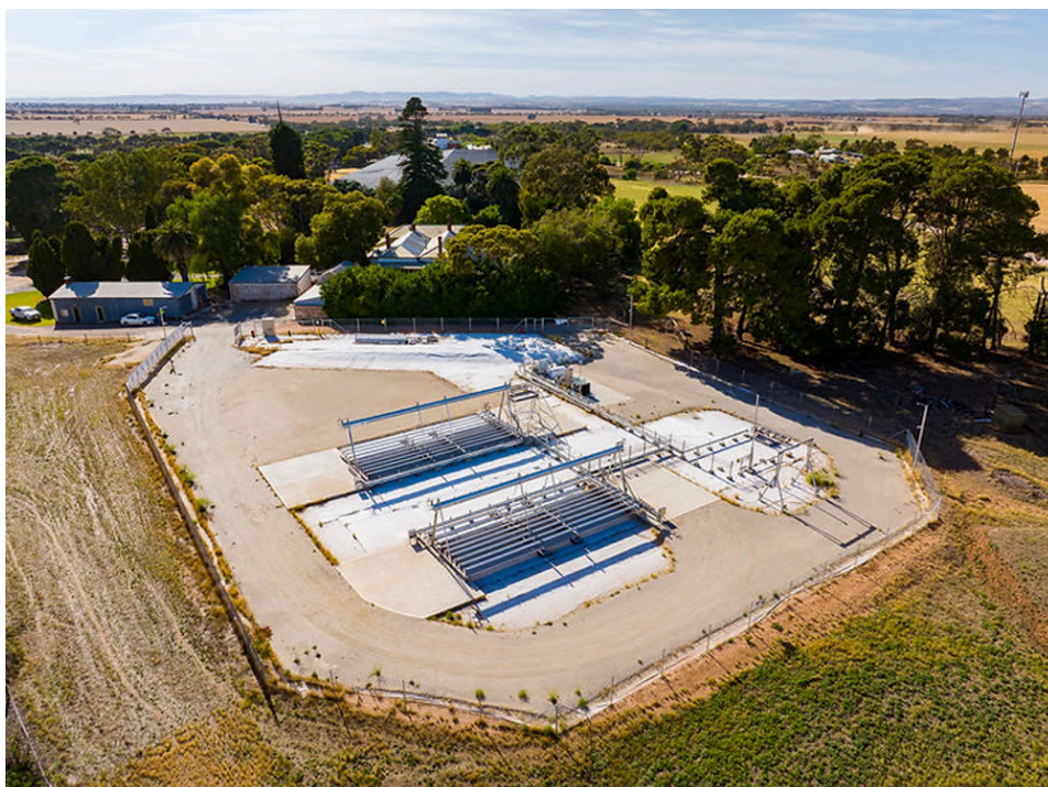
The SPARC Hydrogen Advanced Research Pilot (SHARP) Plant at Roseworthy Campus
